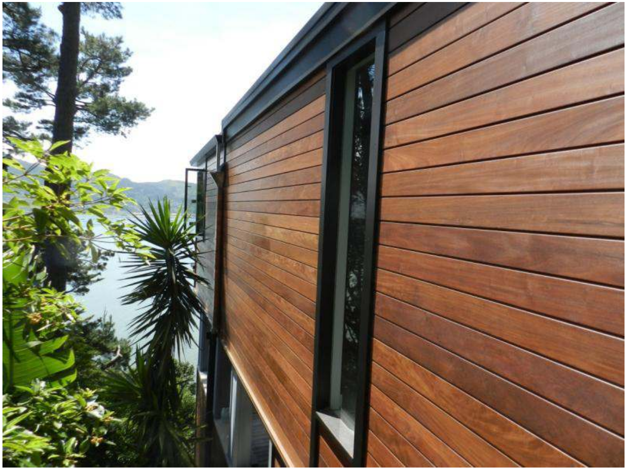
1x6 Ipe rain screen cladding
