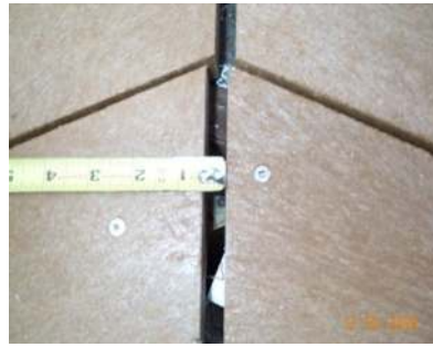
Plastic decking expansion/contraction
