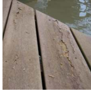
"Composite decking" delaminating and showing deterioration
