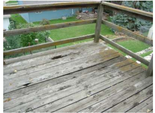
Red Cedar decking exhibiting "dry rot"
