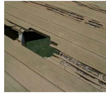
"Hollow" synthetic decking deterioration
