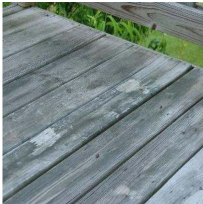
Cupping, checking, mold and mildew
