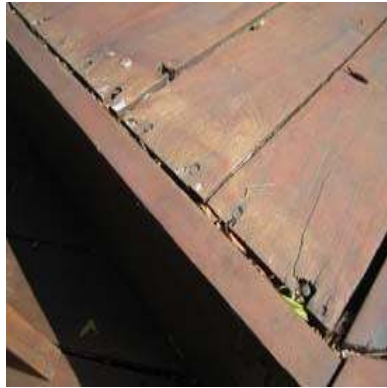
Red cedar decking rotting from moisture
