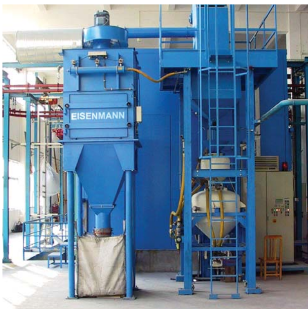
Fig. 1: Shot blasting plant for boiler pretreatment
