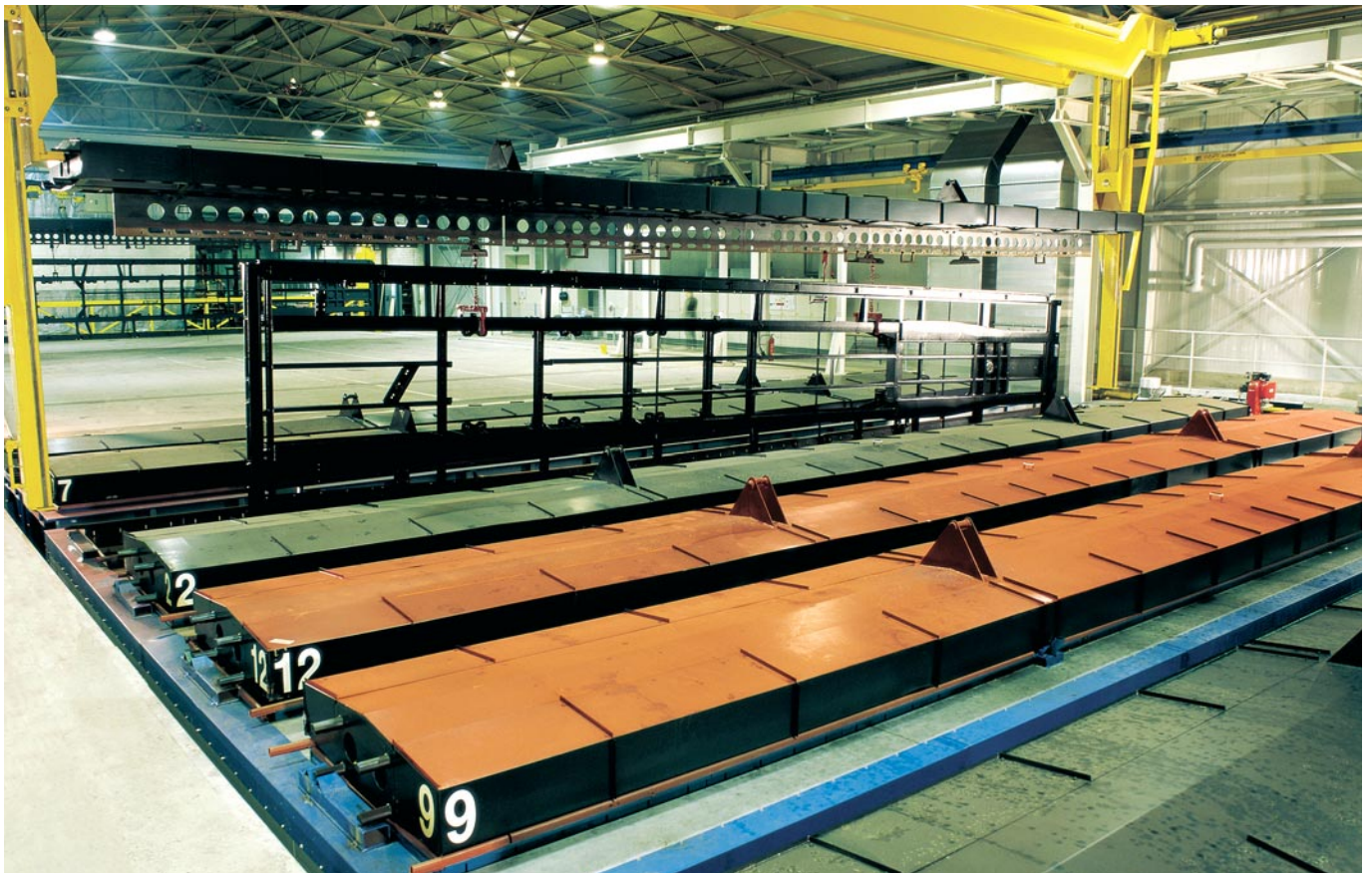
Programmable hoist systems are especially useful for large workpieces with relatively low production volumes such as the truck frames in a dip painting line as shown.
