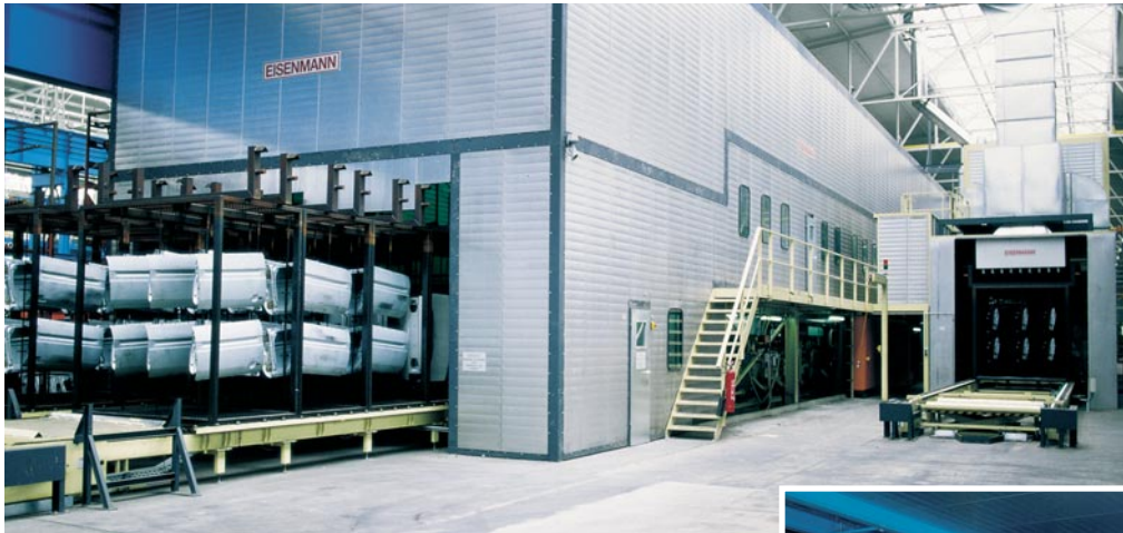
Picture left: Cathodic top coat curing oven with bottom entry/exit for heat loss prevention.
