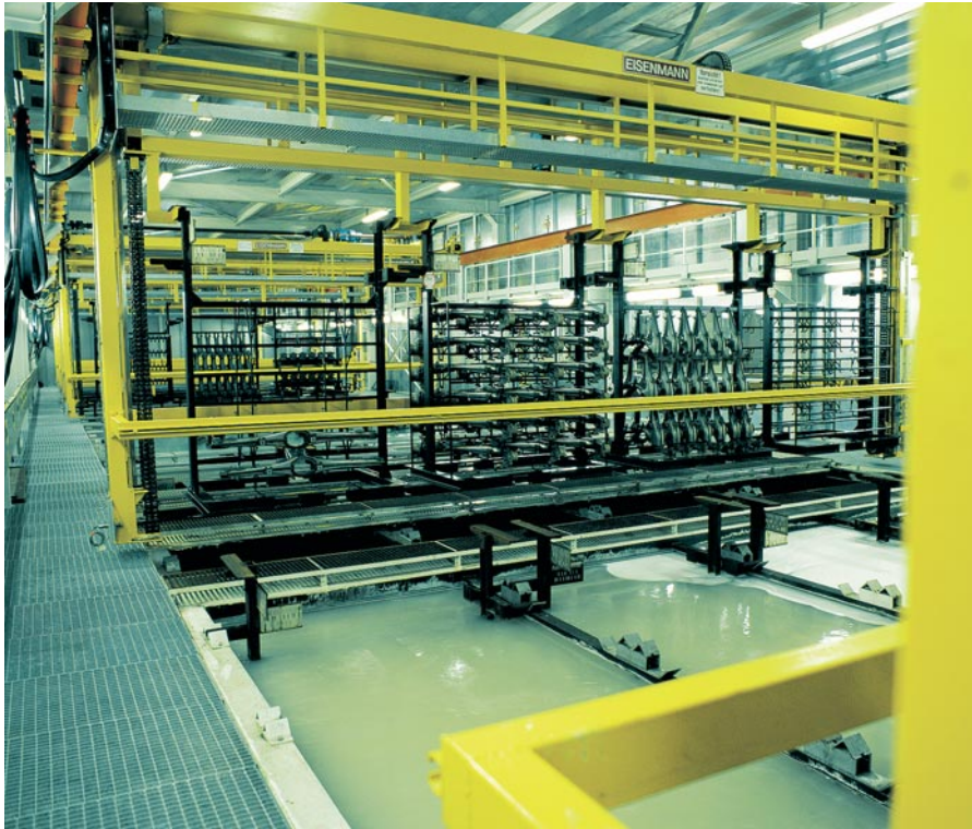
Cathodic E-coat with programmable hoist for automotive components.
