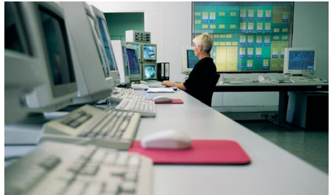
Control center for an automotive paint line.
