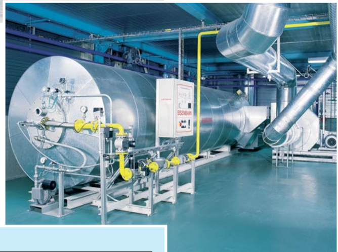
Picture above: Thermal oxidizer with heat recovery for purifying exhaust air from the E-coat curing oven.
