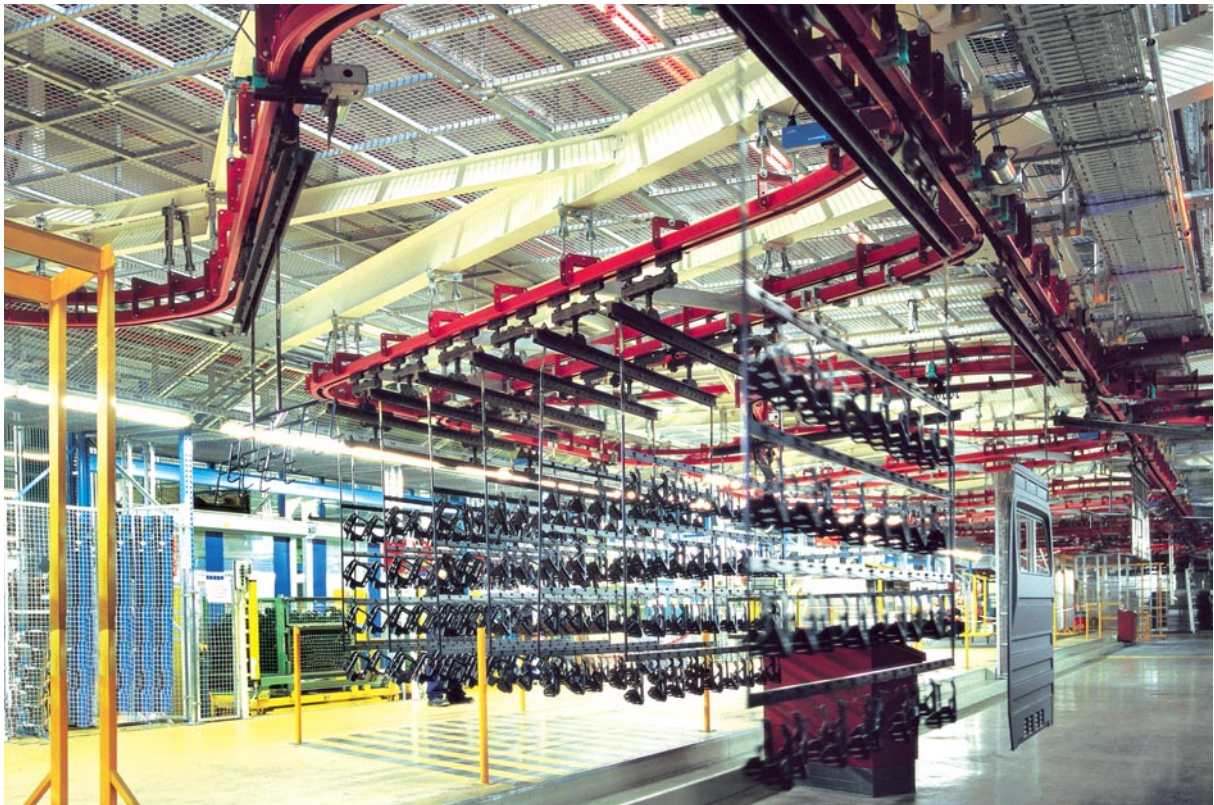
Complex Power & Free conveyor system with numerous pick-up stations, interim storage and process destinations in the automotive industry
