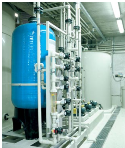
Water treatment system for the extraction of 100% desalinated processing water
