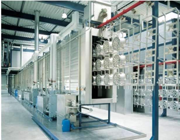
Pretreatment system as part of a powder coating line for wheels
