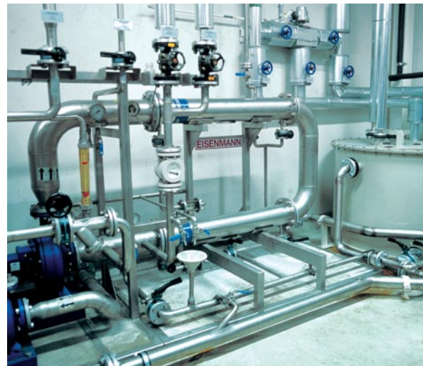
Ultrafiltration for the controlled circulation of degreasing baths
