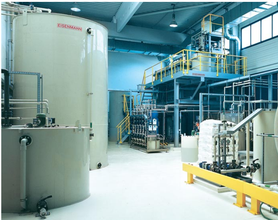
Complete wastewater disposal facility for metal processing, including dip-coating line
