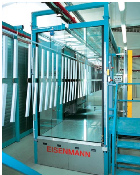
Glass booth at a powder-coating line for switch gear cabinet parts
