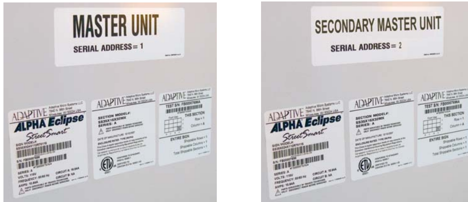
Figure 30. Master/Secondary Master labels
