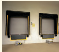
Rolling Service Doors
