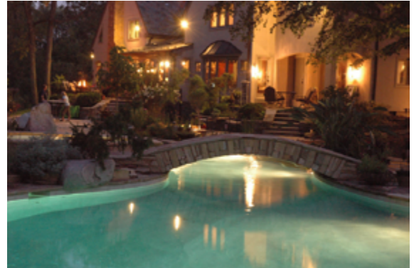
Flood lights installed on this home provide general lighting for the garden and dining area. Sconces illuminate the entryways and uplights accent trees and bushes. The pool has lights that provide ambient lighting in the waters. There is also a lamp-post on the patio.
