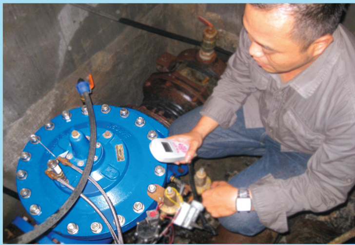
Malang City staff personnel testing the new Singer Valve S106-2PR-BT
