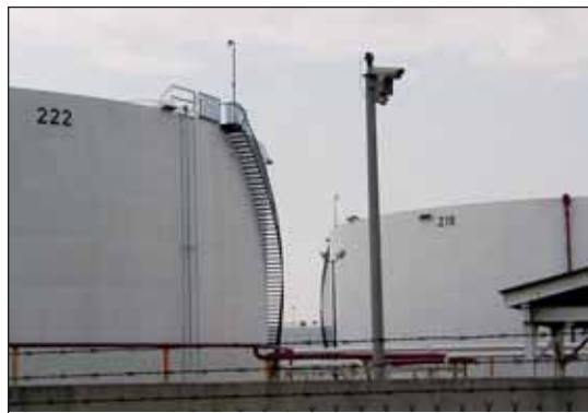
The PTZ camera is part of the perimeter protection for this entire oil depot provided by Sabre Integrated Security Systems LLC, New York.
