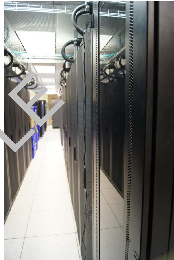
Hot Aisle Example with Return Air Grilles Directly Overhead (Note Hanging Temperature Sensor Array)
