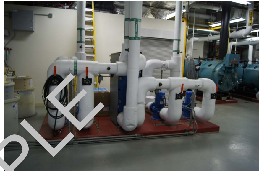
Existing Plate & Frame Heat Exchanger with Dedicated Pumps
