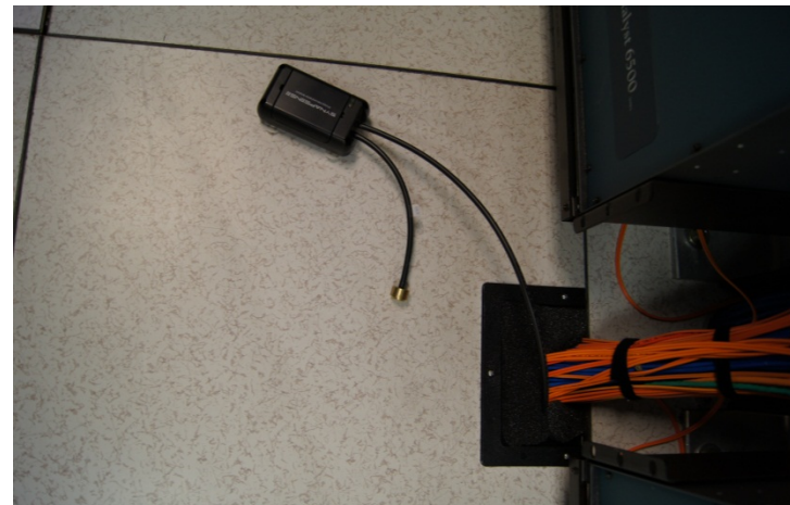
Differential Pressure Node Resting on Floor, with Sensor Above and Below Raised Floor Surface
