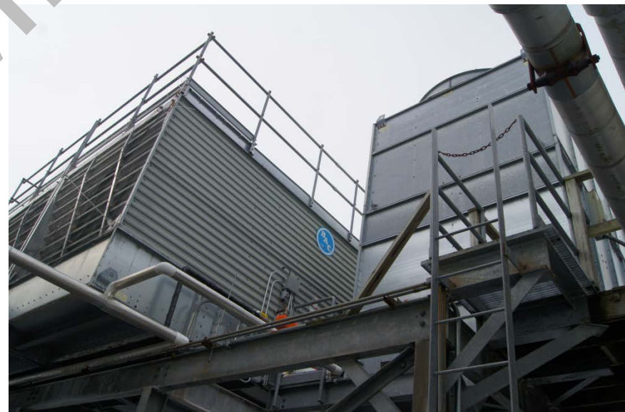
Dedicated Cooling Tower for Free Cooling Heat Exchanger
