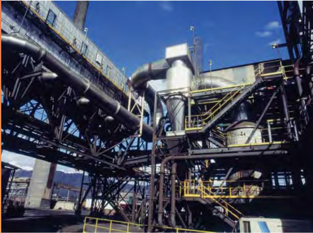
Fluid Bed Dryer Used for Copper Concentrate
