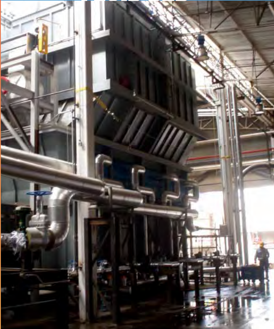
Fluid Bed Dryer for Waste Biomass Product
