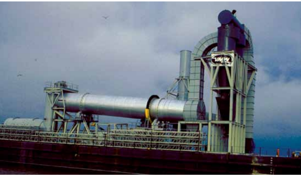
Barge-Mounted, Mobile Rotary Dryer Used to Process Bauxite
