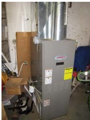
Forced Air Heating System
