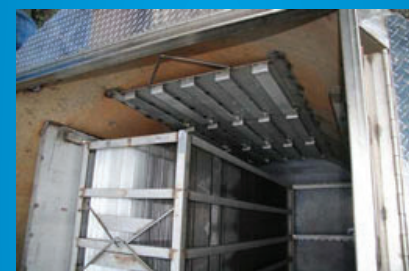
The Multi-Pack in Concrete API Pit
