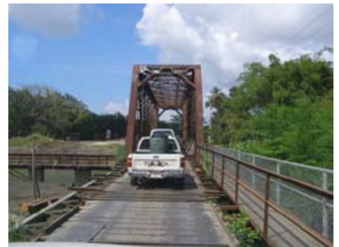
New bridge taking form next to old one lane bridge in Parrita
