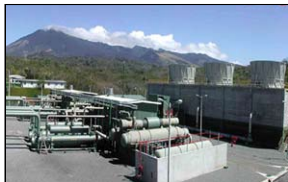
Miravalles Geothermal Plant
