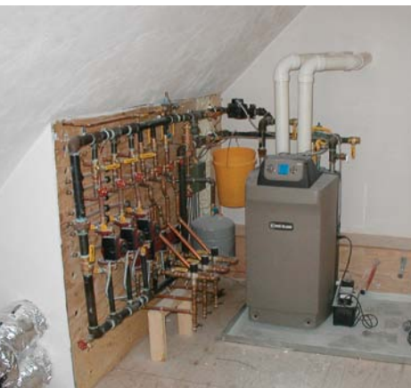
Radiant heat is fueled by a 98.6% efficient Weil-McLain modulating gas boiler ( www.weil-mclain.com ). Cast-iron piping is used wherever possible to limit PVC use.
