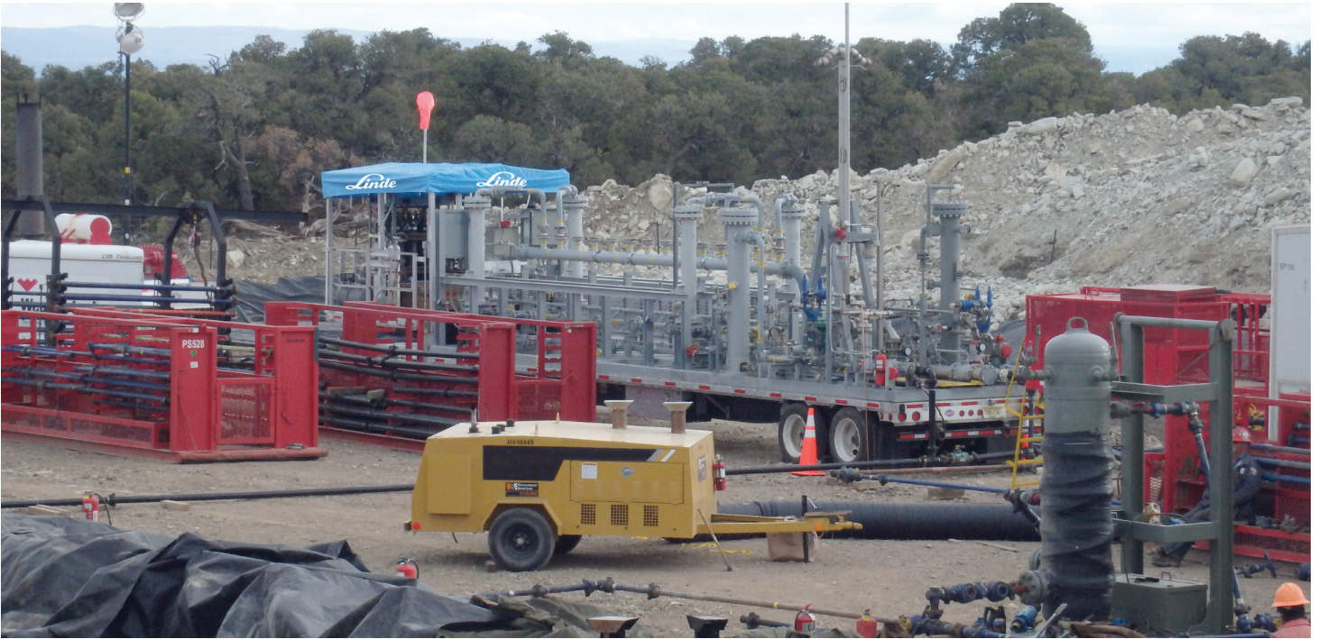
Image 1: New Linde Mobile Gas Clean-up Unit (MGCU) for scrubbing CO 2 out of early flowback gas.
