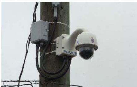
AutoDome cameras are mounted on streetlamp poles in areas where incidents are likely to occur.
