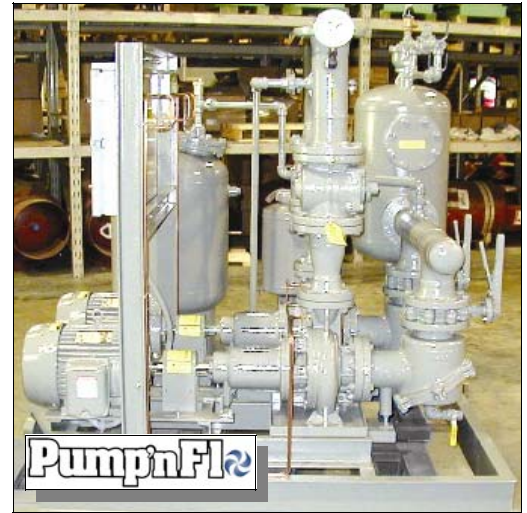
One of two duplex chilled water pumping packages complete with air control, pump accessories, and control panel
