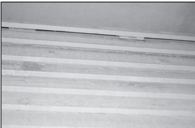
Figure 222. This is similar to figure 221. The top-most spacer is cut to not lay on the siding, but over the existing furring and insect screen. One stand-off is probably more than adequate.
