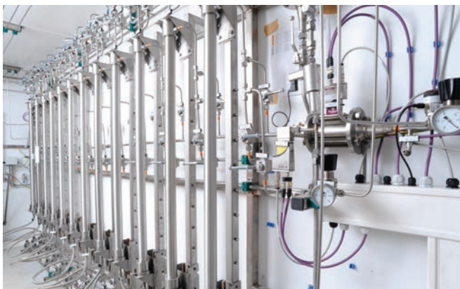
The heart of the biogas upgrading plant: membrane technology is a feasible option for upgrading biogas and a promising area for the future.
