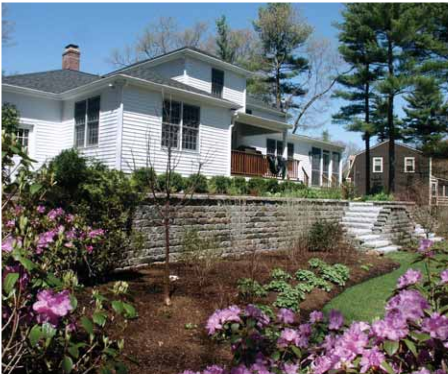
This segmented retaining wall was installed to replace a failing railroad tie wall. Granite switchback steps with paver landings were used to break up the steep grade change.
