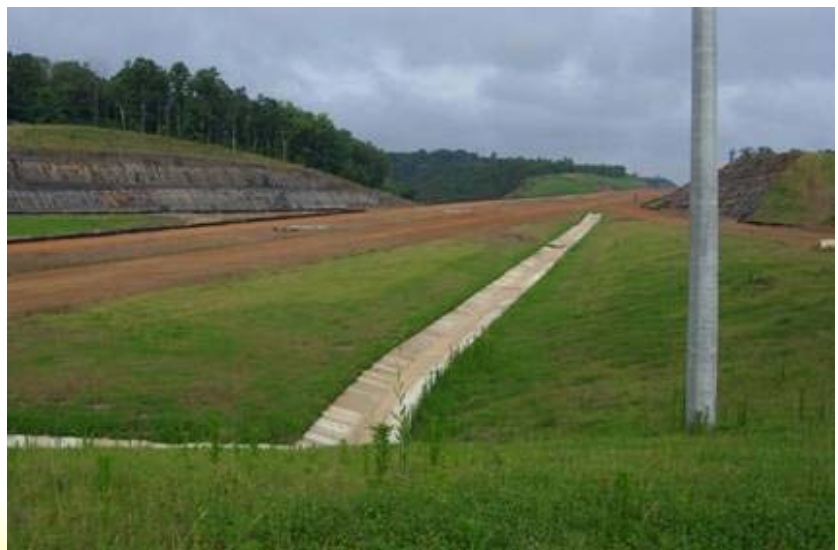
The new road bed lay erosion free for 6 month using APS 740 Silt Stop powder
