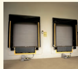
Rolling Service Doors
