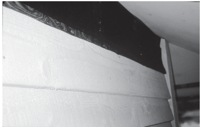
Figure 220. This figure indicates a sequential step from figure 218. The battens have been carried up to the soffit. As the finished siding approaches the top of the wall a single or double vent can be used. The choice is only determined by the desired “look” and/or performance. Only experience will tell how much ventilation is necessary or appropriate. Cut a strip of fiberglass insect screen to be stapled to the top leading edge for the last “common” siding course above the reveal line of the existing course of siding. This sequence is then followed by using cutoffs of the furring material. Use 1/2 inch pressure treated plywood, ripped to a width of 2 7/8 inches. A wide strip is used to increase the width of the nailing base. Keep the nails at least 1 inch away from any end of a board to decrease the likelihood of splitting the siding.
