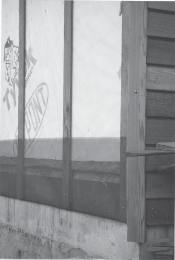
Figure 219. Shows the installation of insect-proof mesh vent screening installed over the bottom opening of the ventilated wall. This allows air and water drainage to easily occur behind the exterior rain-shield sheathing.
