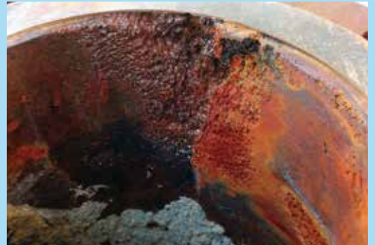
Visible damage from cavitation prior to Singer Valve
