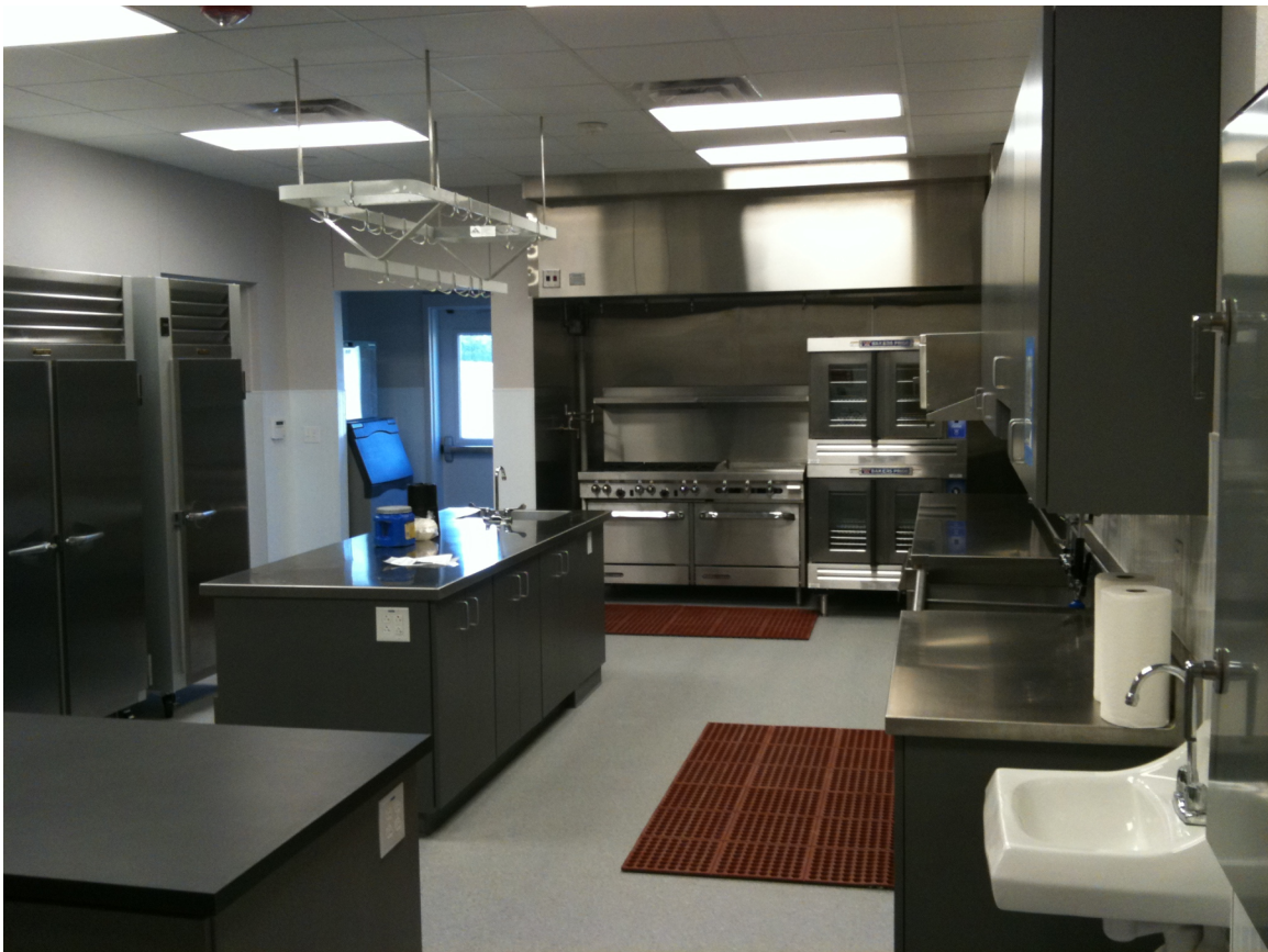
Full Commercial Kitchen. Note: hand sink is used as accessible sink Foundation United Methodist Church, Temple TX
