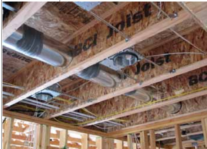
Running ductwork and trunk lines through the web brings the entire system into conditioned airspace.
