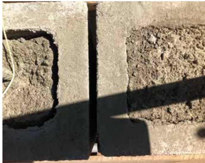
Solid Center. Concrete masonry blocks are filled to create enough mass to mitigate indoor temperature swings.
