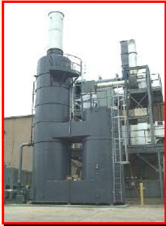
Photo is a QUADRANT SR-15,000 Silicone Series Thermal (recuperative) Oxidizer designed, Manufactured and installed by Catalytic Products International, Inc.
