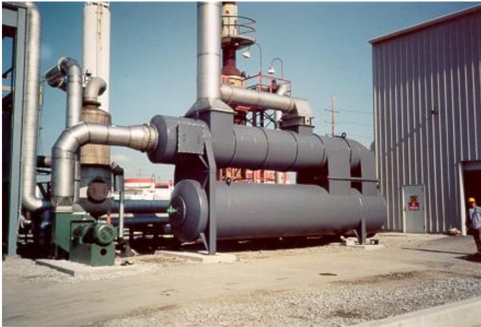
Photo is a QUADRANT SR-7,000 Thermal (recuperative) Oxidizer designed, manufactured and installed by Catalytic Products International, Inc.
