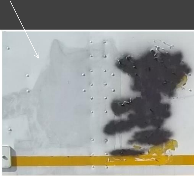
Graffiti and other vandalism
