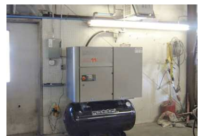
The shop's old air compressor was loud and starting to leak oil, so Owner Dana Cooper researched Mattei and made the move to the company's rotary vane compressors
