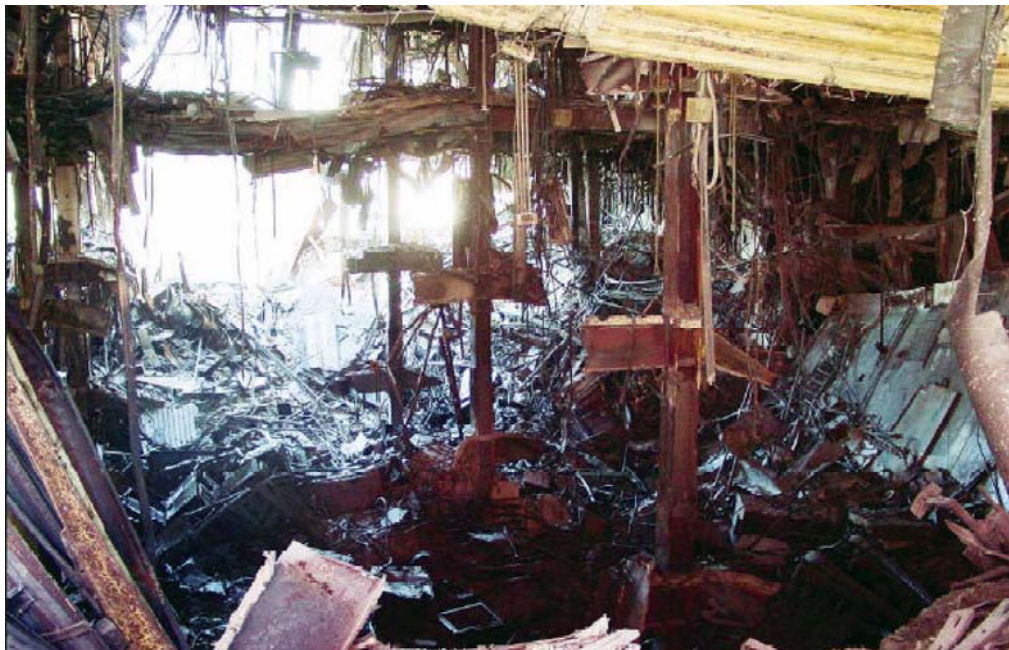
Figure 2. Internal Collapse Area in WTC 5 (World Trade..., 2002).
