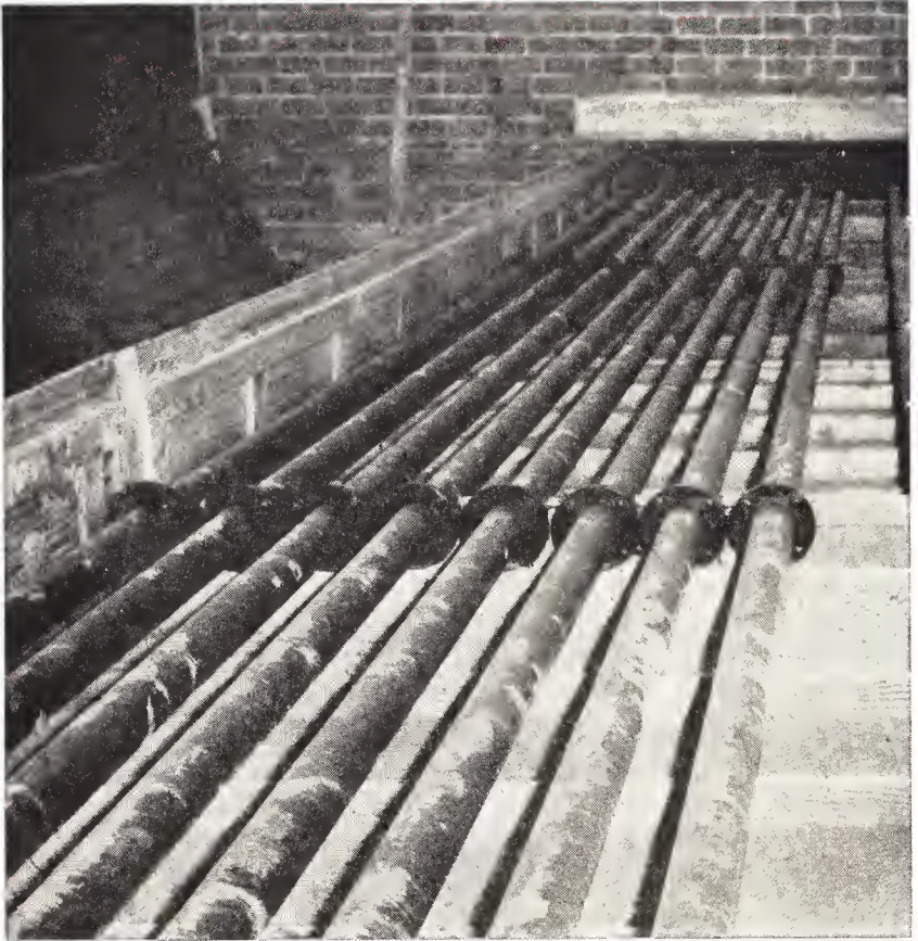
Cast iron pipe carries hot corrosive liquid in chemical plant
