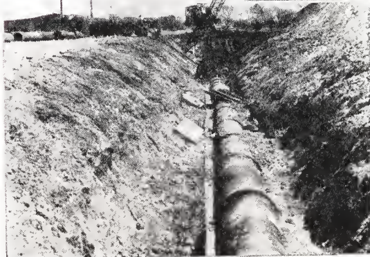
Mechanical joint cast iron pipe being installed for a deep sewer line.
