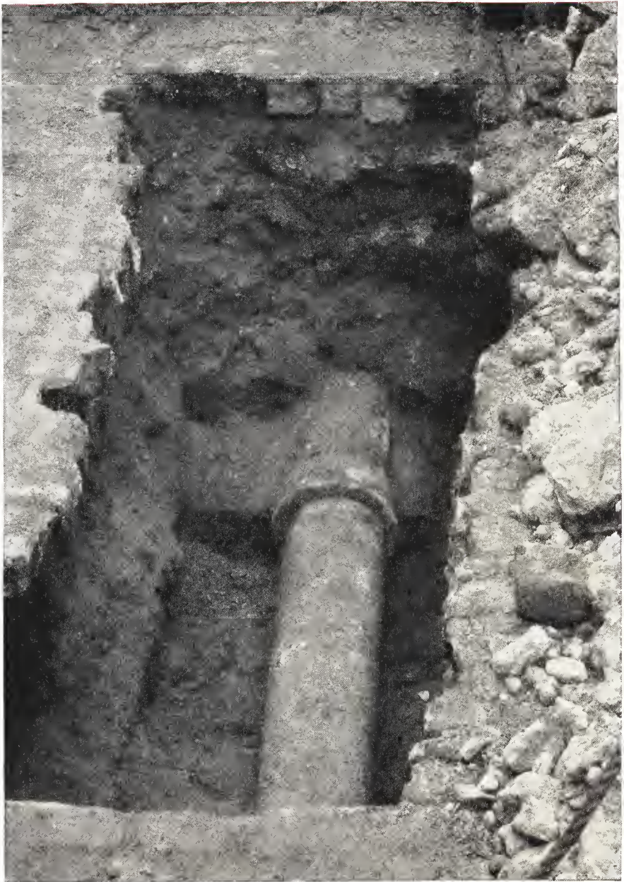
America's oldest cast iron gas main, laid in Baltimore in 1834
