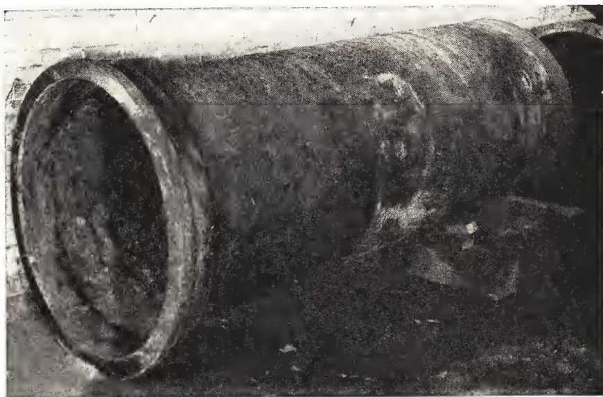
New York, N. Y. Removing a 36-inch cast iron water main from tunnel in Highbridge. Installed in 1848 to carry water from Cratan Aqueduct across Harlem River and abandoned when bridge was reconstructed. Sold as scrap.
