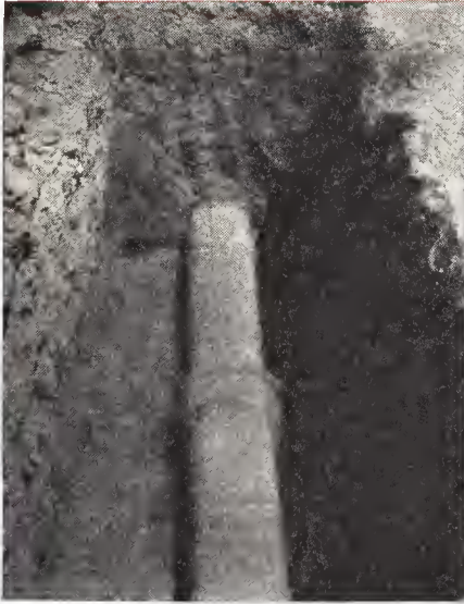
Richmond, Va. A section of a cast iron water main, salvaged and relaid of 88 years of age, uncovered for inspection in its 113th year of service to the taxpayers of Richmond, Va.
