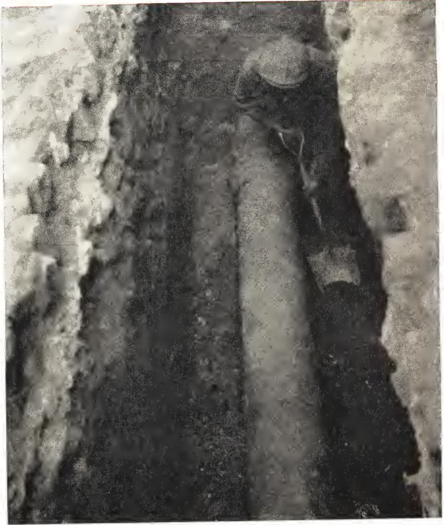
America's oldest cast iron water main, laid in Philadelphia in 1821
