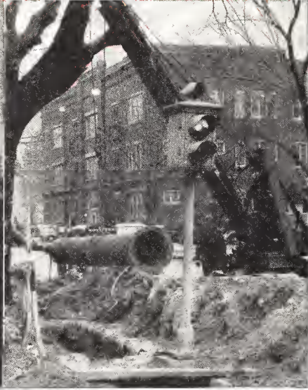
Kenasha, Wis. Removing a 14-inch cast iron water main for replacement with new 24-inch cast iron pipe. After 43 years' service, the old 14-inch pipe proved to be in excellent condition and was relaid in another section of the city.
