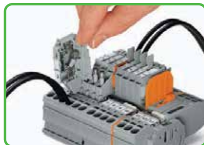
Opening the cover to replace the fuse.
