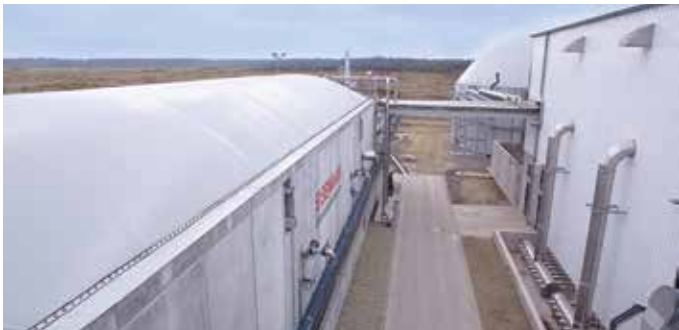
Concrete digester with a capacity of 900 m 3 .
