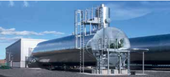
A 340 m 3 steel digester with external sanitization in a 160 m 3 cylindrical steel tank.
