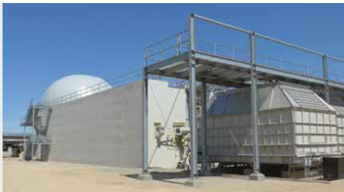
Material intake and digester.
