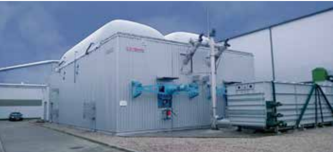
Concrete digester with a volume of 2 x 800 m³.
