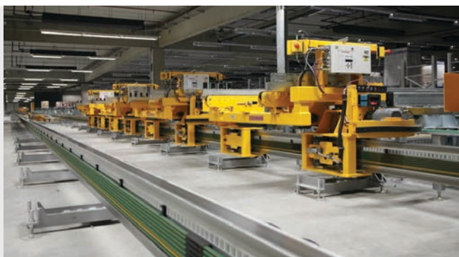
Smart solution: the IEMS conserves resources and reduces costs as there is no need for a steel structure.
