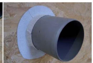
Completely sealed opening
