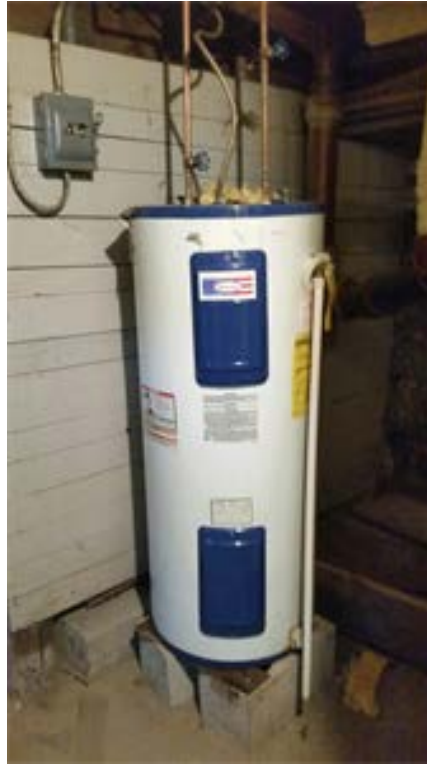
Hot Water Tank
