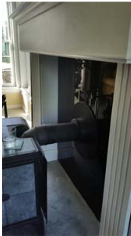
Stove Pipe Connection to Wall
