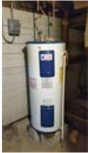
Hot Water Tank
