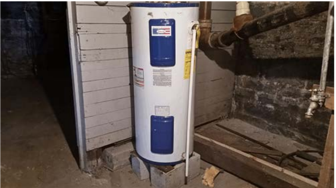
Hot Water Tank
