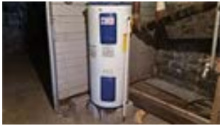
Hot Water Tank
