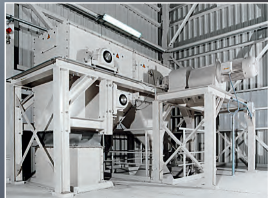
Discharge Section of a WB 640 Conveyor with 30 kW (40 HP) Drive
