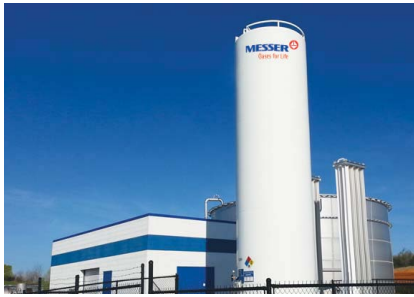
The plant's 6,000-gal liquid oxygen tank
