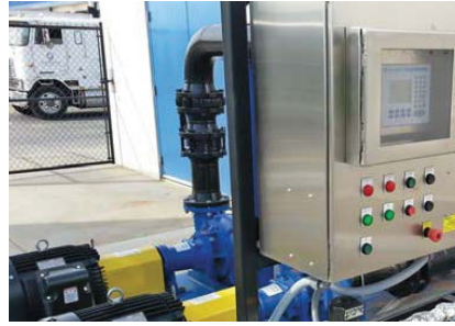
Control panel moderating appropriate oxygen flow
