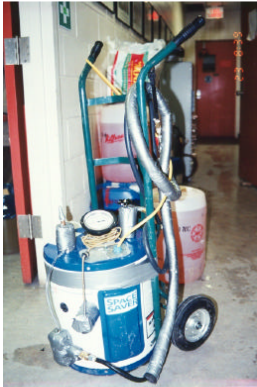
Photo 3.12 Hot Water Tank
