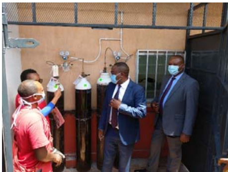
Commissioning of the Oxygen Gas Manifold at the Machakos Level 5 Emergency Department by the Machakos County CEC for Health, Dr Ancent Kituku
