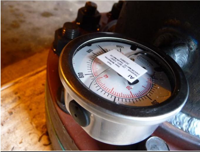
Figure 15 – Hydro Test Gauge.
