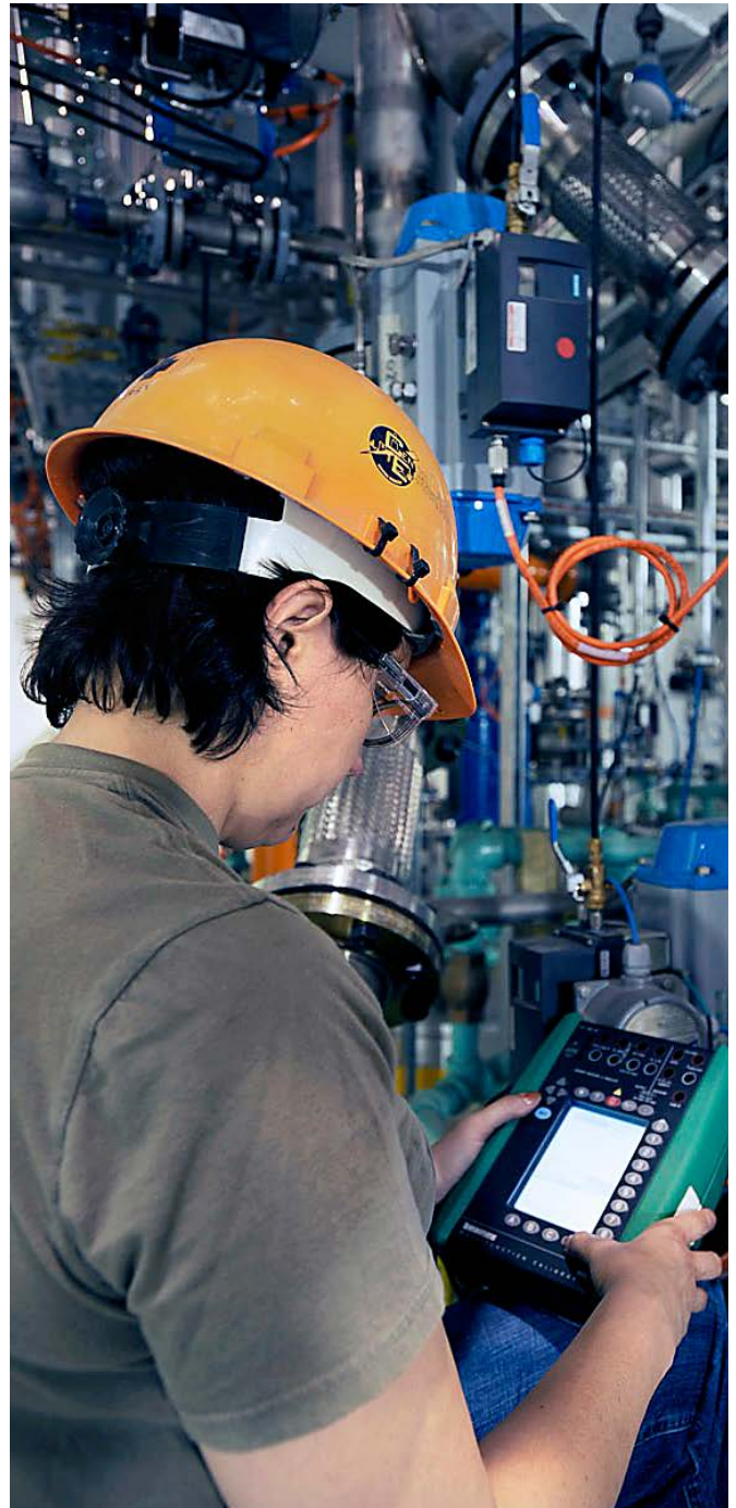
Marcella Dupuis, Project Engineer, uses an MC5 to calibrate one of 3,300 PROFIBUS PA devices.
