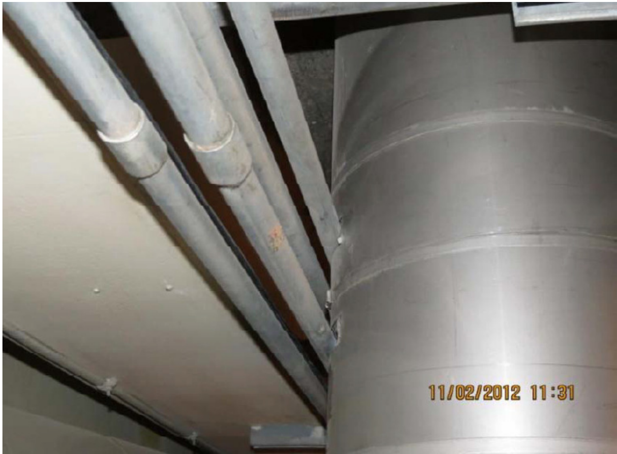
Figure 1 Interesting Cable conduit hot pipe separation
