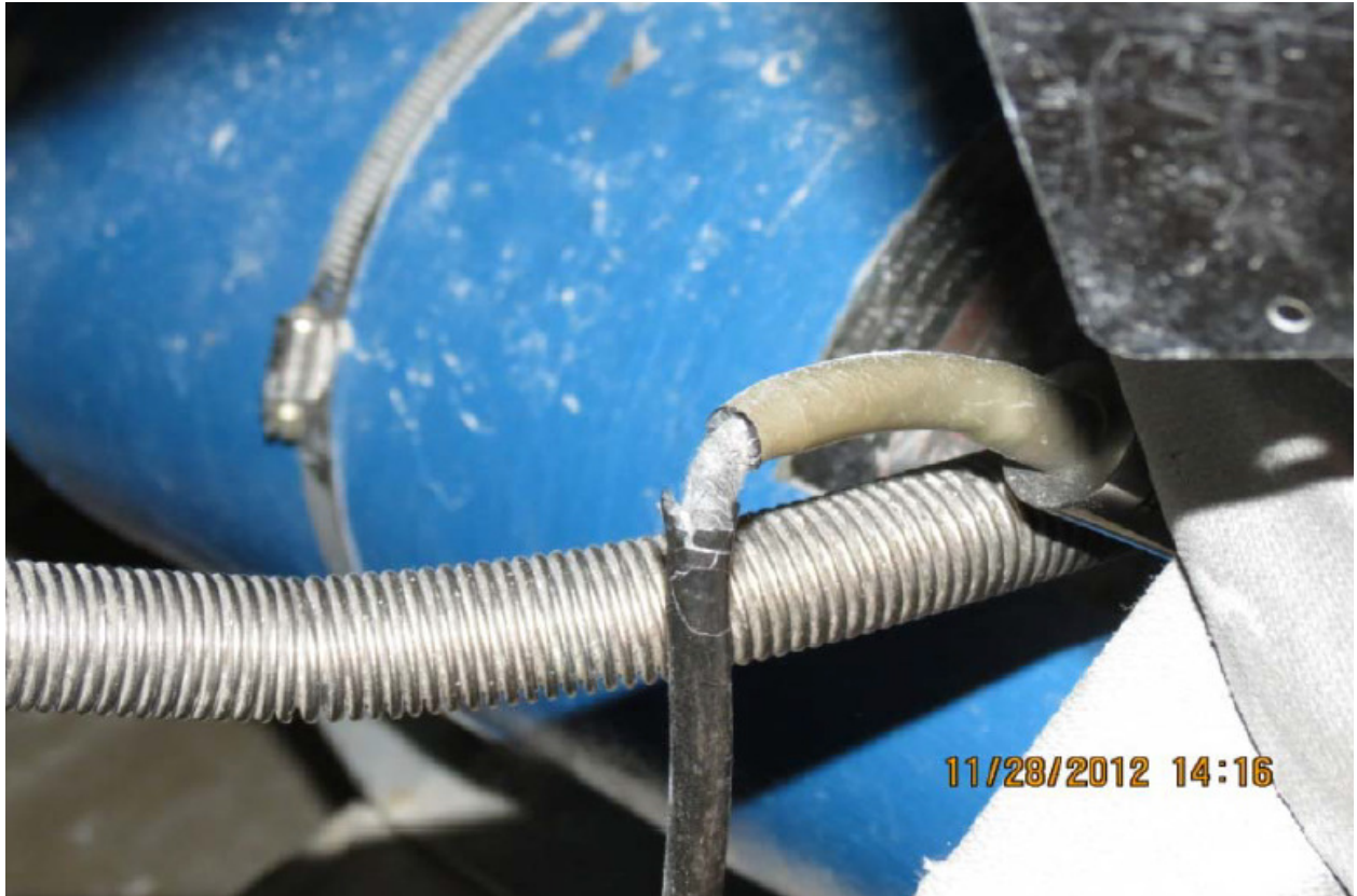
Figure 2 Thermally Degraded Cable Jacket
